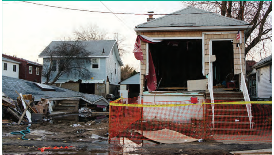
Figure 3: Damaged homes in New York City as a result of Hurricane Sandy, November 2012. Photo by Somayya Ali Ibrahim.
